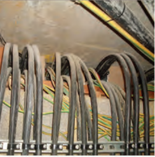
Power cables penetrating a compartment floor with no penetration seal installed (incorrect). Courtesy of Sharpfibre Ltd.
