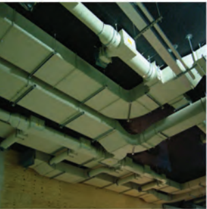
Installations of fire resisting ductwork. Courtesy of StGobain Isover (top) and Fire Protection Ltd (bottom)
