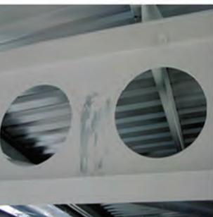
Slumping of intumescent paint on a cellular beam. Courtesy of Exova Warringtonfire Ltd.
