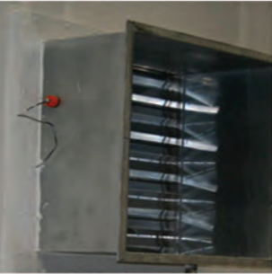
Fire damper correctly installed in the plane of the wall with no damage to the penetration seal. Courtesy of Paul White.
