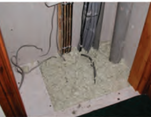
Incorrect use of 'foam' as a penetration seal. Courtesy of Siderise Ltd.
