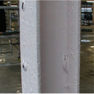
Degraded intumescent paint. Courtesy of Exova Warringtonfire.
