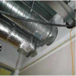
In this installation, the dampers are not in the plane of the wall, the duct is not protected and it is unlikely that the dampers have been tested in a cellular beam. Courtesy of Paul White.
