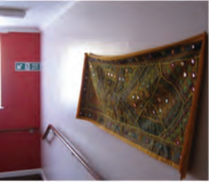
Flammable carpet on a wall can assist fire spread. Courtesy of Graham Fieldhouse.
