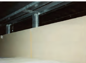
Vertical compartmentation not extending up to floor slab above (incorrect). Courtesy of Exova Warringtonfire.
