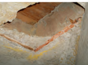
Compartment floor with a hole passing through to the laminate floor in the flat above (incorrect). Courtesy of Sharpfibre Ltd.
