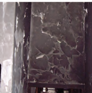
Delaminated paint that has burned in a fire. Courtesy of Exova Warringtonfire.
