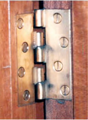
Worn hinges allow door to drop. Courtesy of Jacky Sinclair.
